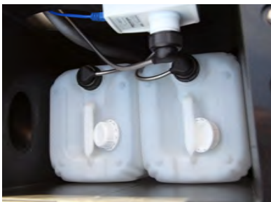
methanol storage for fuel cell operation
