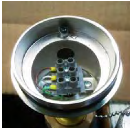
Typical Gems flow switch fitted with large 240V junction box
